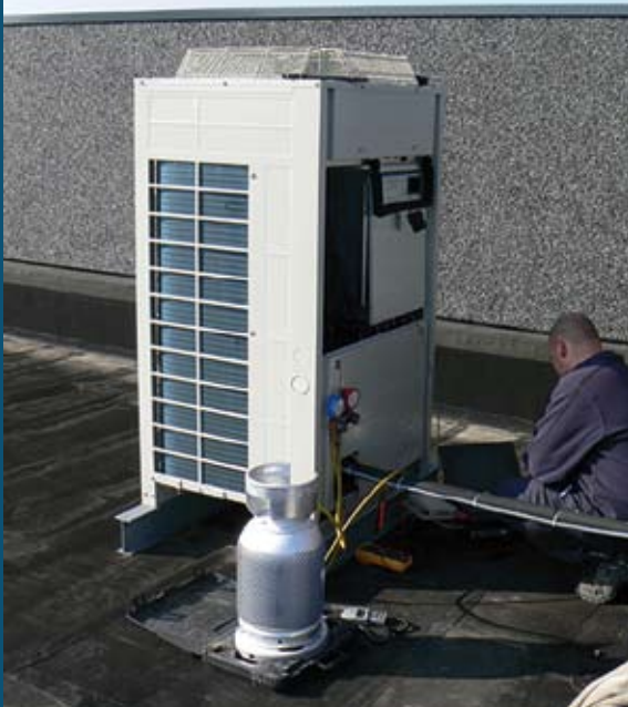
➤ Daikin A/C Belgium technician inspects refrigerant charge during maintenance.
